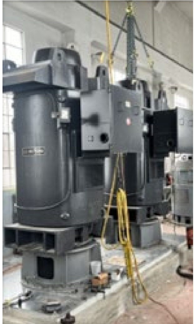
Portneuf Pumping Plant at Fort Hall Indian Irrigation Project, Idaho
