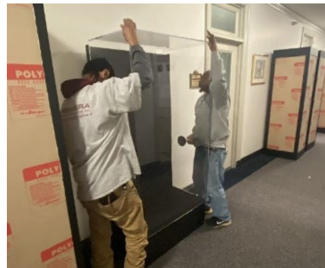
Photo. New Era contractors assisting with installing new museum-quality exhibit cases in BIA hallway, Corridor 4600.
