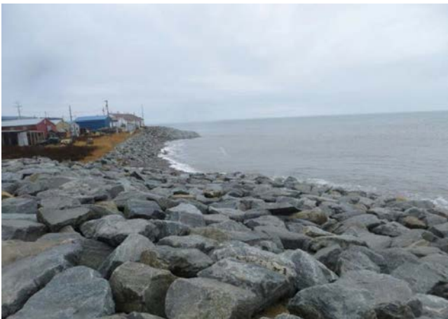
Erosion by Alaskan Village
