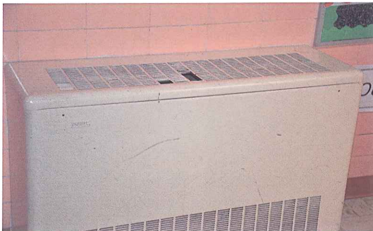
Location: Elementary School Building 431 Backlog No.: N36-08-431-M-004-1 Deficiency: Outmoded radiator heater and malfunctioning during adverse weather condition
