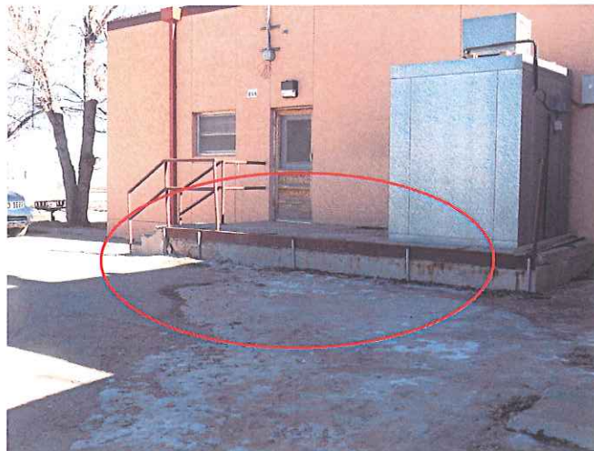
Location: Cafeteria/Dining Hall Building 434 Backlog No.: N36-08-434-M-040-1 Deficiency: Loading dock area cracked and heaving. Water ponding on pavement creating safety hazard
