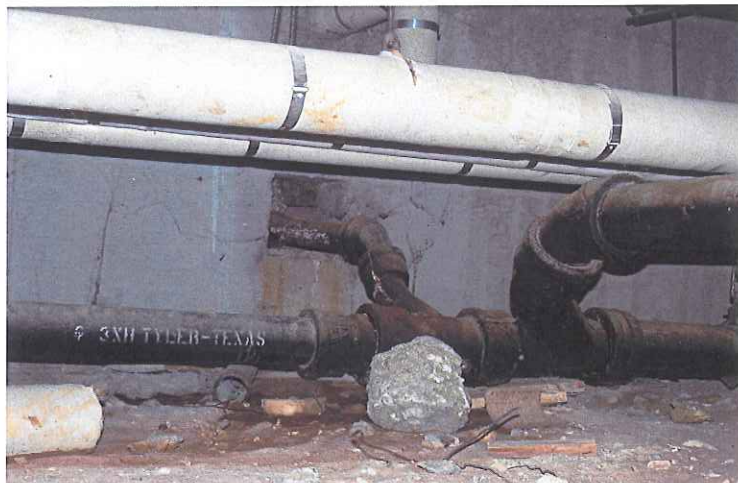
Location: Secondary School Building 432 Backlog No.: N36-08-432-M-023-1 Deficiency: Outdated wastewater fixtures creating ongoing maintenance and does not comply with Uniform Plumbing Code
