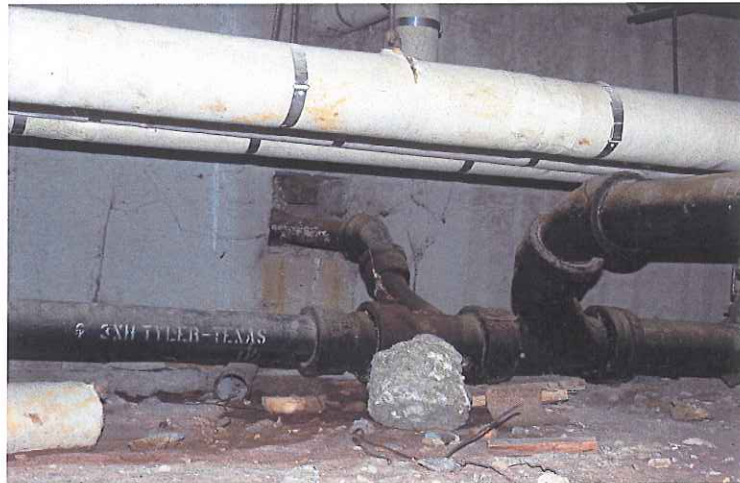
Location: Elementary School Building 431 Backlog No.: N36-08-431-M-040-1 Deficiency: Outdated wastewater fixtures creating ongoing maintenance and does not comply with Uniform Plumbing Code
