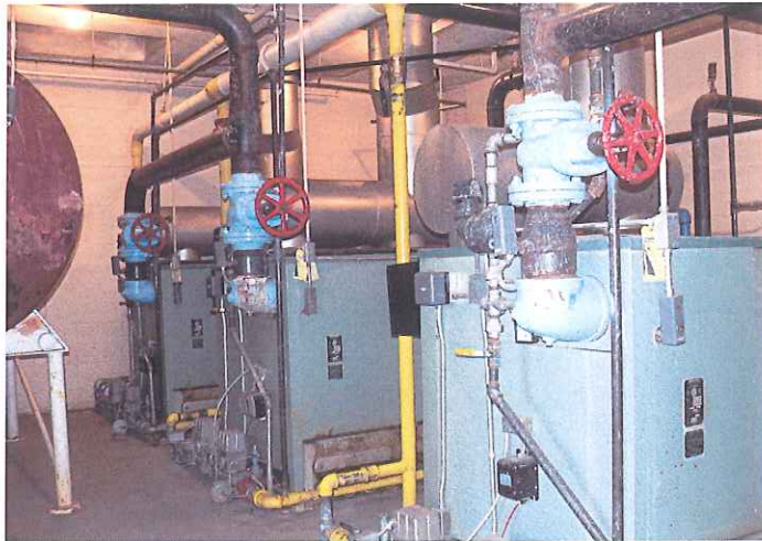
Location: Residential Building 436 Backlog No.: N36-08-436-M-042-1 Deficiency: Boilers for hydronic heating systems are in poor condition with only minimal temperature controls
