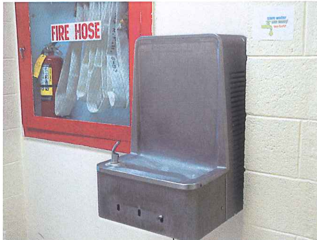
Location: Residential Building 436 Backlog No.: N36-08-436-M-047-1 Deficiency: Outdated water foundation system does not comply with ADA (Violation of BIA Handbook 1.2(D))
