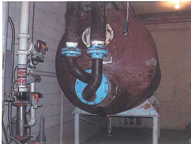
Location: Residential Building 436 Emergency Repairs: Storage tank got rust corroded which caused plumbing system to malfunction and required expensive emergency repairs
