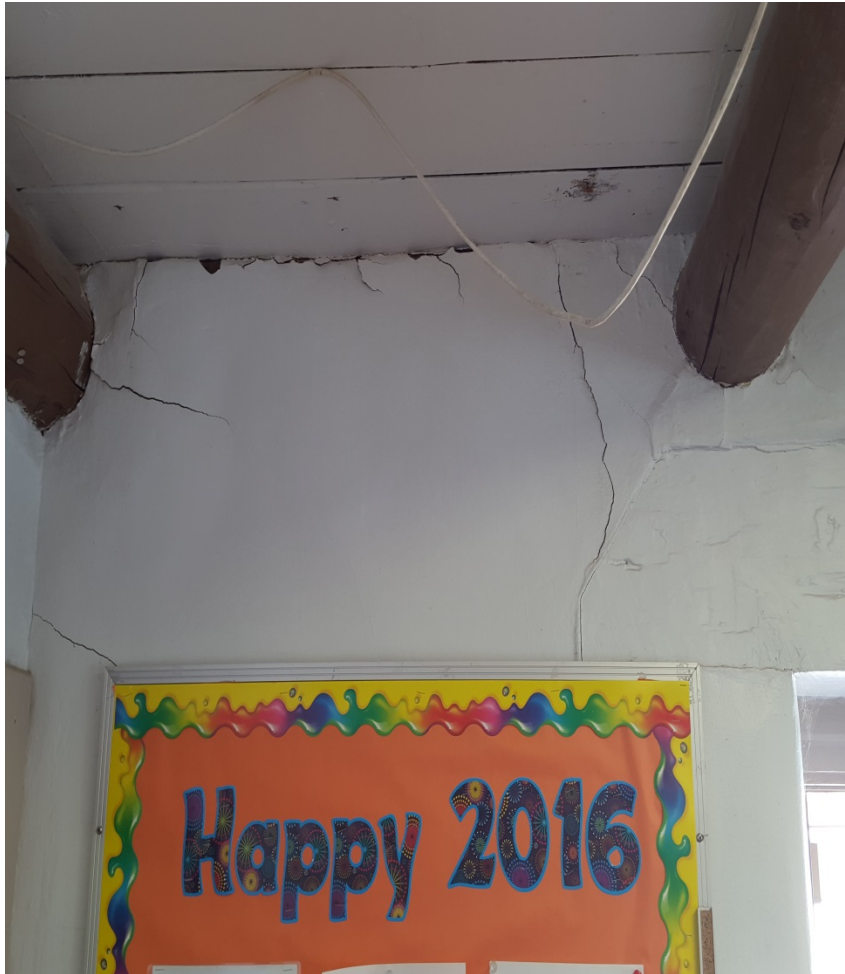
Cracks on the Main Office Walls and Computer Cables Hanging Down
