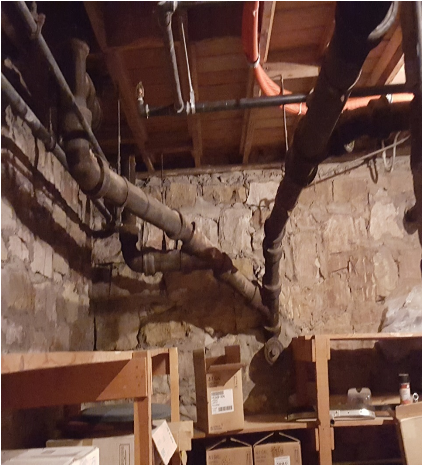
Foundation Walls that Holds Up the Main Building are Cracking & Waste Water Pipes from Bathrooms are Antiquated
