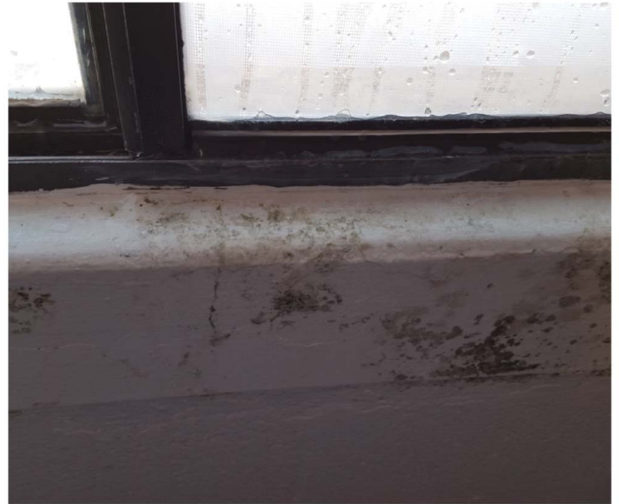
Condensation from Double-pane Window; Dripping and Icing-up; Causing Mold Buildup on Cinderblock Wall in Quarters
