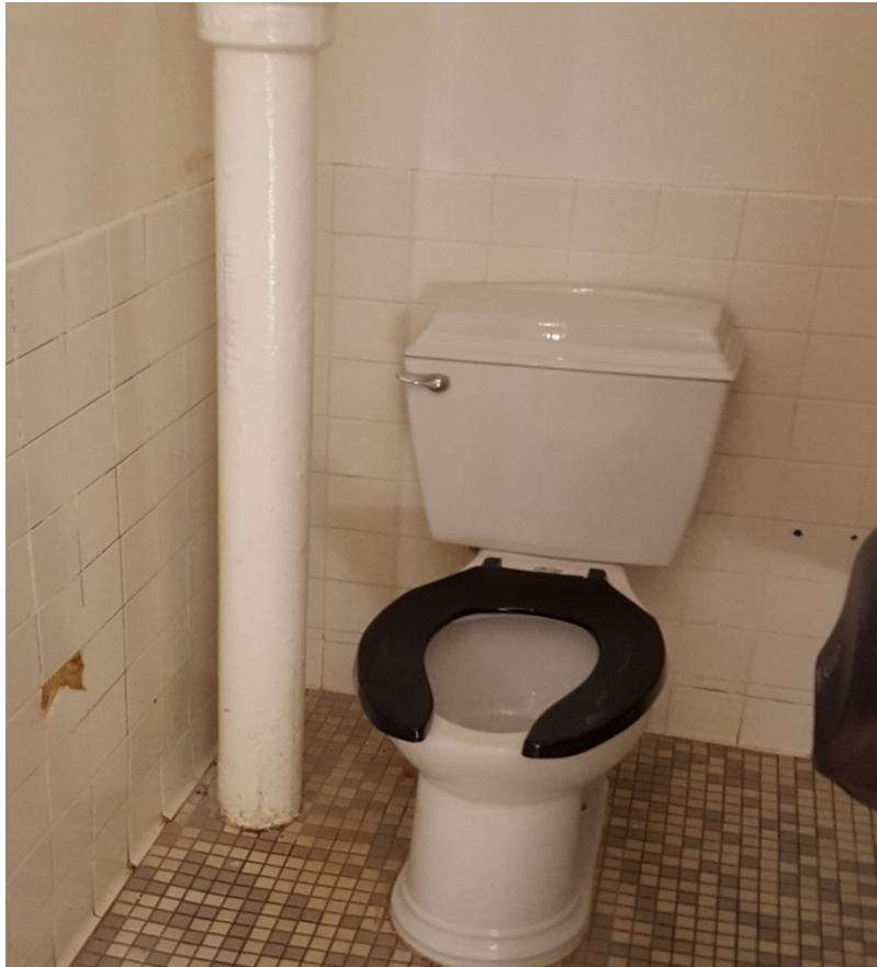
Only One Commode in the Boys Bathroom in Main Building
