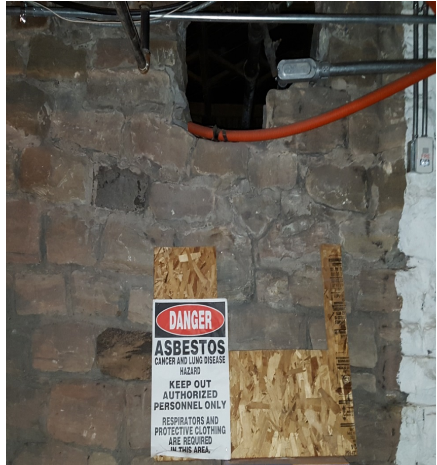
One of Two Crawlspace to get to Utility Pipes and Conduits Underneath the East Side of the Main Building
