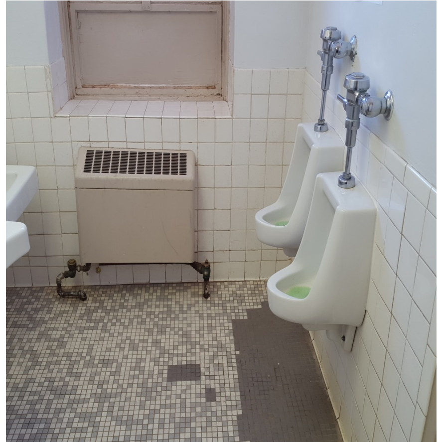
Only Two Urinals in the Boys Bathroom in Main Building
