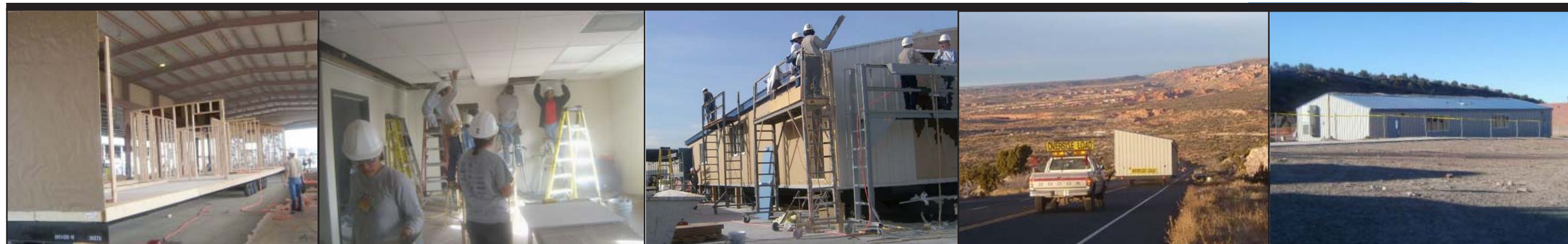
Construction of the special modular classroom took place at Modular Solutions in Ehrenix, Ariz. It was then transported to the Navajo Reservation and set up next to the Nazlini Community School building, which is near Ganado, Ariz. The BIA school serves students in grades K-8.
