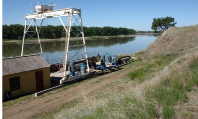
Frazer Pumping Plant, Ft. Peck Irrigation Project, MT
