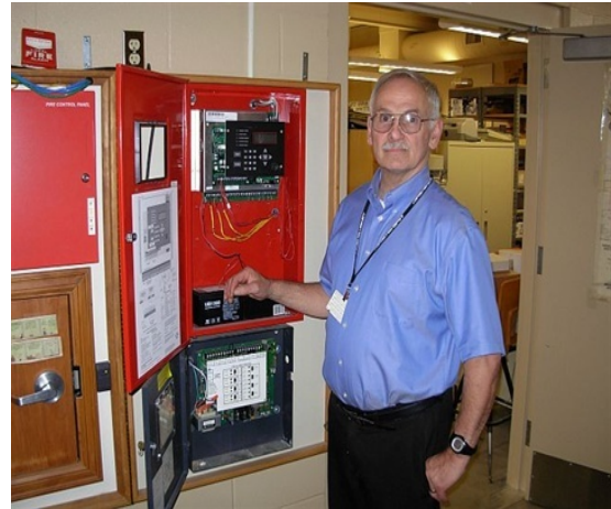
Testing the fire alarm system
