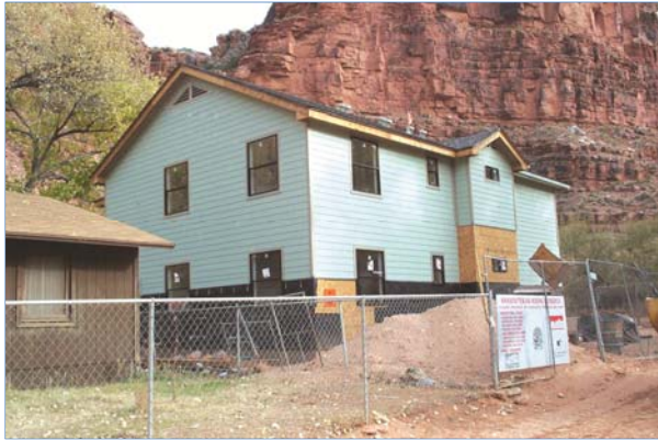
Quarters under construction in Supai village at the bottom of the Grand Canyon in Arizona.
