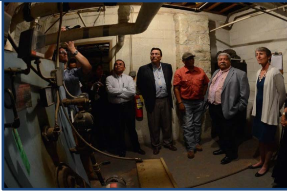
Secretary Jewell is shown an outdated and often broken boiler located in a converted coal chute at Crystal Boarding School in New Mexico. The room is cloaked in asbestos and this makes repairs to the boiler extremely difficult.
