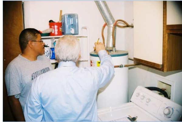
Inspecting a water heater in one of the Quarters at Tohono O’Odham, AZ.
