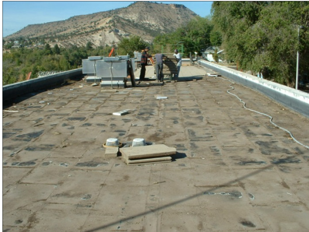
A roof is being repaired at the Warm Springs Detention Center in Oregon
